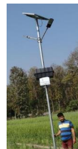
Solar street light
